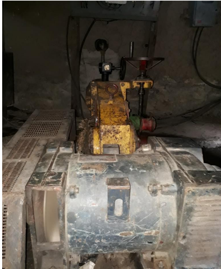
Picture 3: Turbine generator of the project
